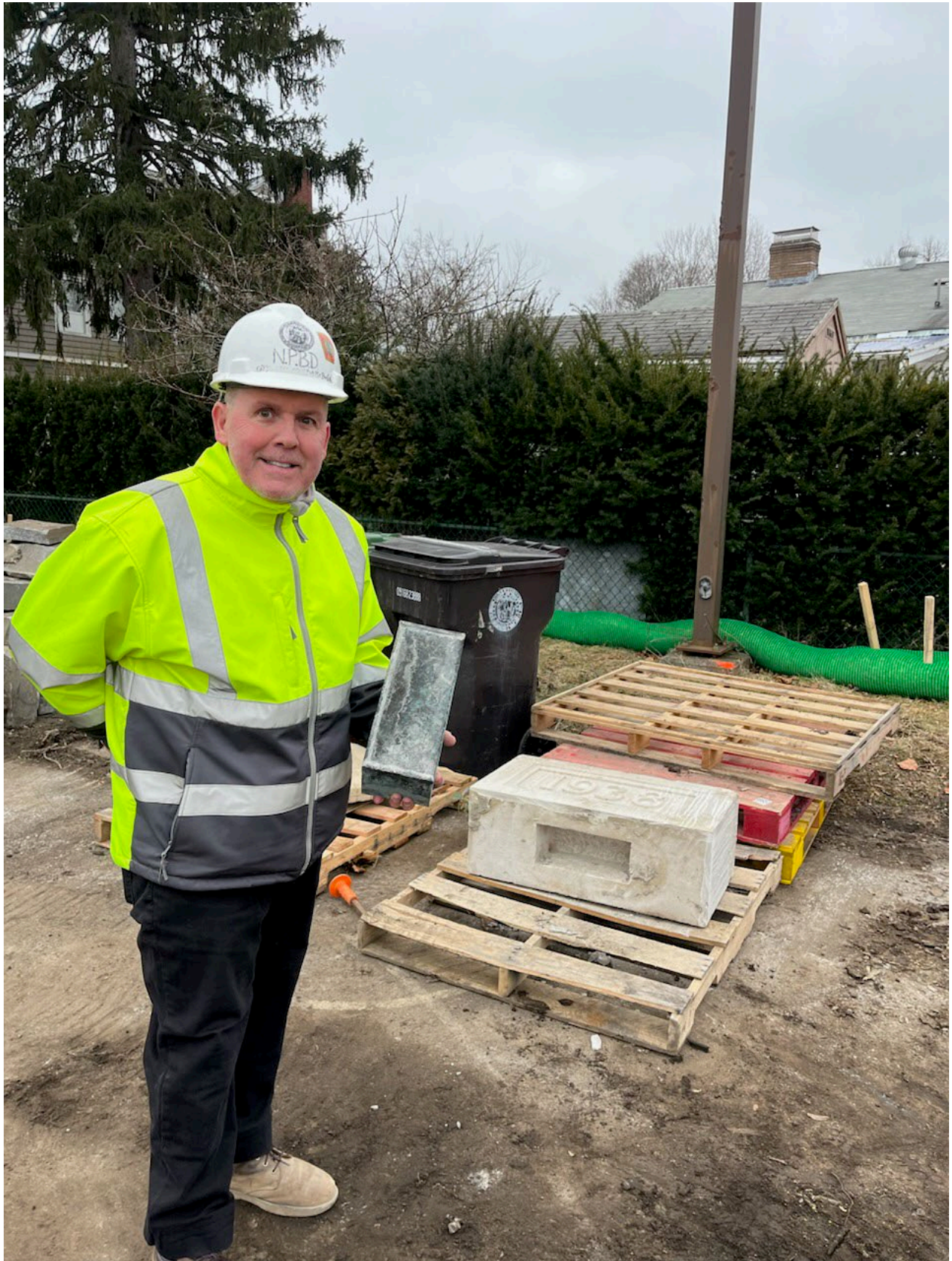
Public Buildings Project Manager Tommy Rooney is seen above with the time capsule from 1938. It was successfully removed and transported to Jackson Homestead for safe keeping until the Groundbreaking event when it will be opened.
