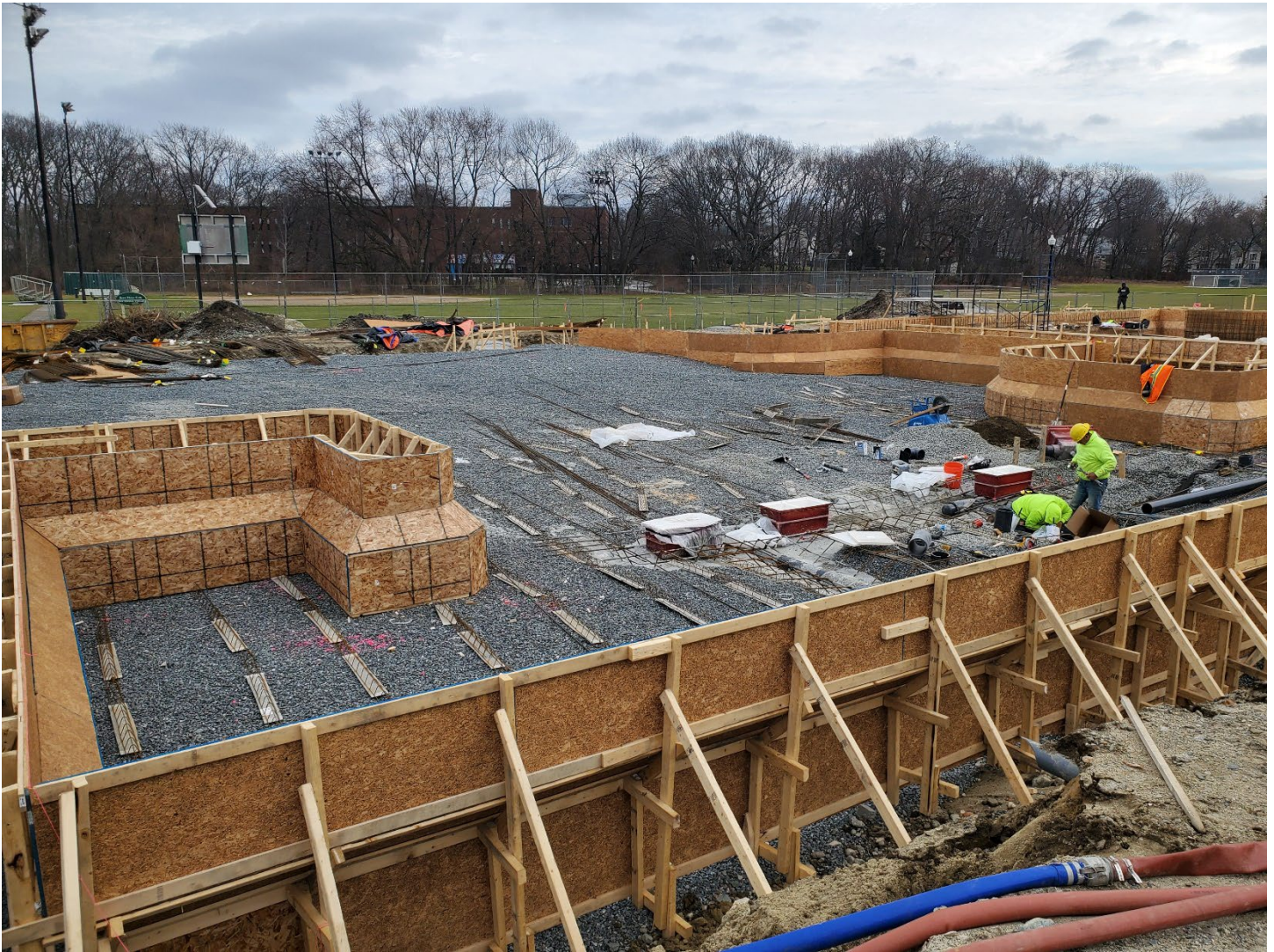
The framing crews are already forming the zero-entry recreational pool. Once the competition pool concrete pours are complete, we'll start pouring concrete for the recreational pool.
