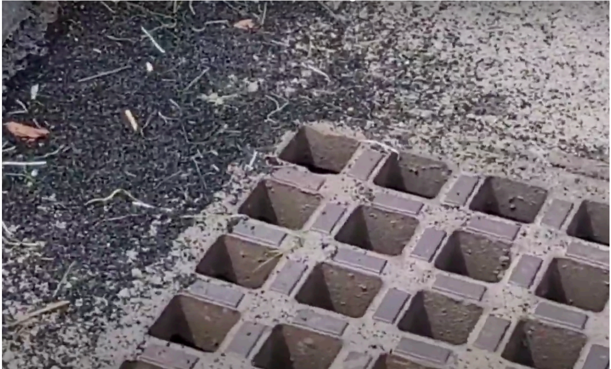
Crumbs of old fill material lying near stormwater drain
