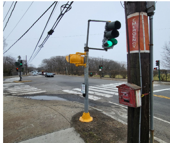
Pictured: Water ponding on the northwest corner of Crafts Street at North Street.
